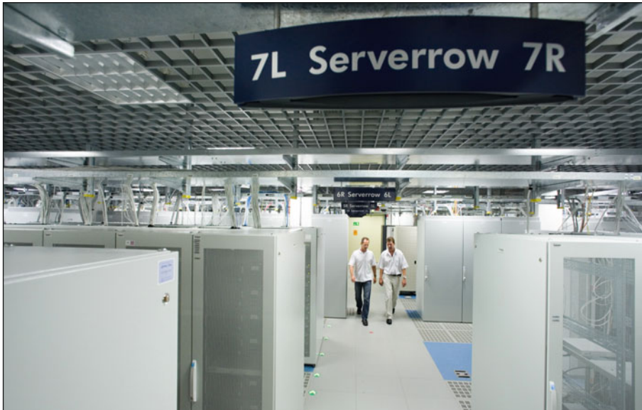
Server room at SAP Hosting, St. Leon-Rot © SAP AG/Wolfram Scheible
